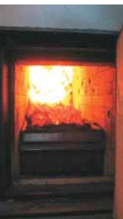
Woodchip boiler Carwood Close Burngreave, Sheffield
